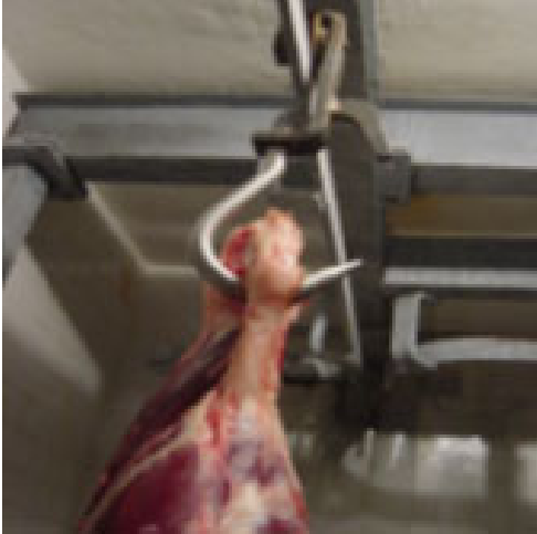
Fig. 481: Adequate material for refrigerated rooms: Overhead galvanized rails and beams, stainless steel meat hook
