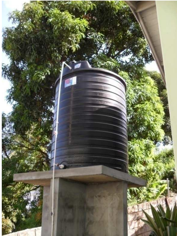
1000 gallon water tank installed at the Lowmans Primary School in St. Vincent and the Grenadines
