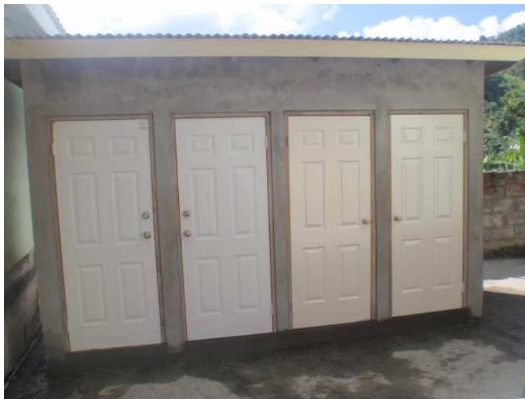
Four (4) shower units constructed at the Lowmans Primary School in St. Vincent and the Grenadines
