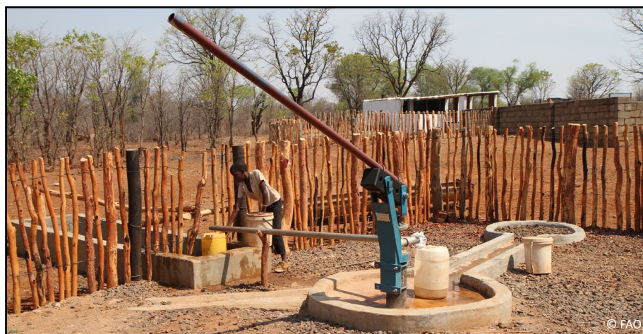
Infrastructure Development: In the foreground is the newly drilled borehole serving both animals and humans and in the background is the rehabilitated diptank in Lupane District
