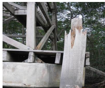
Picture 2 Close-up of Viewing Tower showing damage
