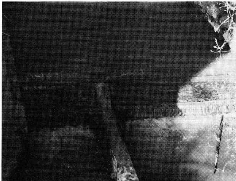
FIGURE 4-1. - Simple fixed proportional flow divisor on small irrigation canal in Cyprus.
