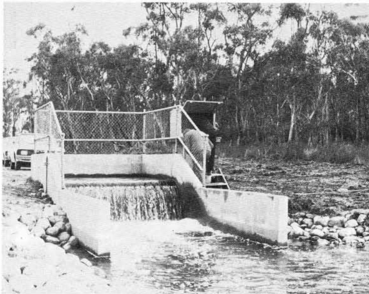
FIGURE 3-35. - Dissipation structure and measuring weir at the pipe outlet. (Discharge 10 \text{ ft}^3/\text{s} .)
