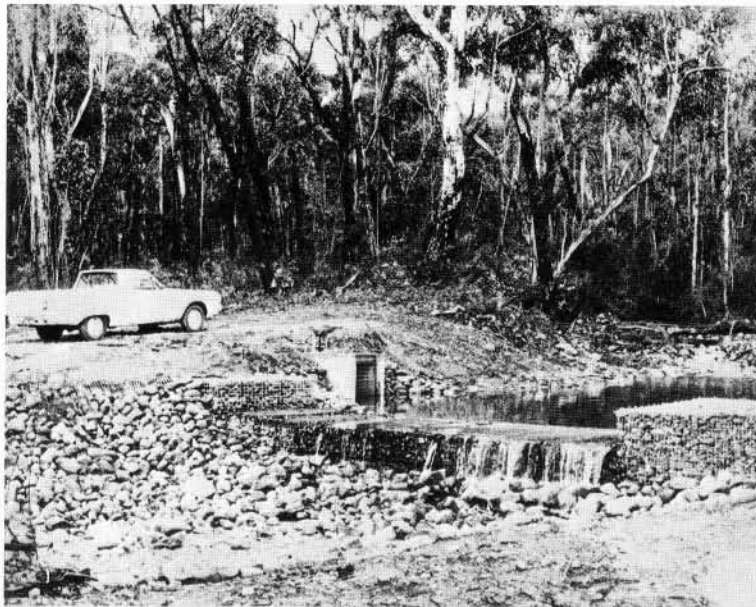
FIGURE 3-32. - General view of the stone mesh weir and inlet box. (Almost all the flow - 12 \text{ ft}^3/\text{s} - is being diverted.)
