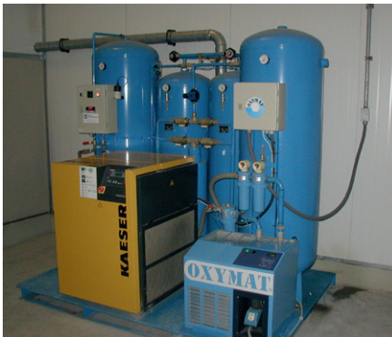
Figure 5.2 Oxygen generator. Control and service of special installations must be taken care of.
