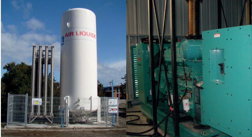
Figure 2.21 Oxygen tank and emergency electrical generator.
