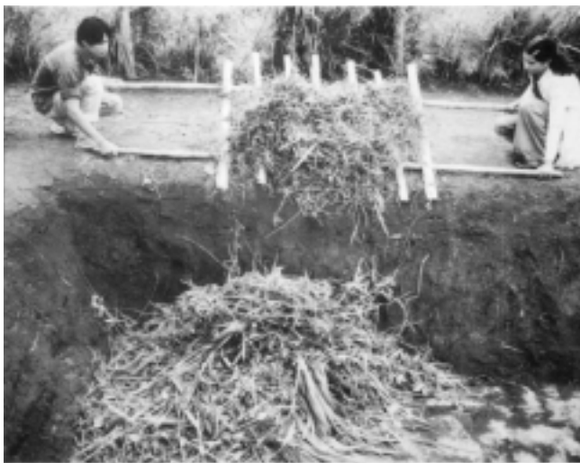
PLATE 1 Tipping organic wastes into a pit; they are spread out into an even layer [FAO]
