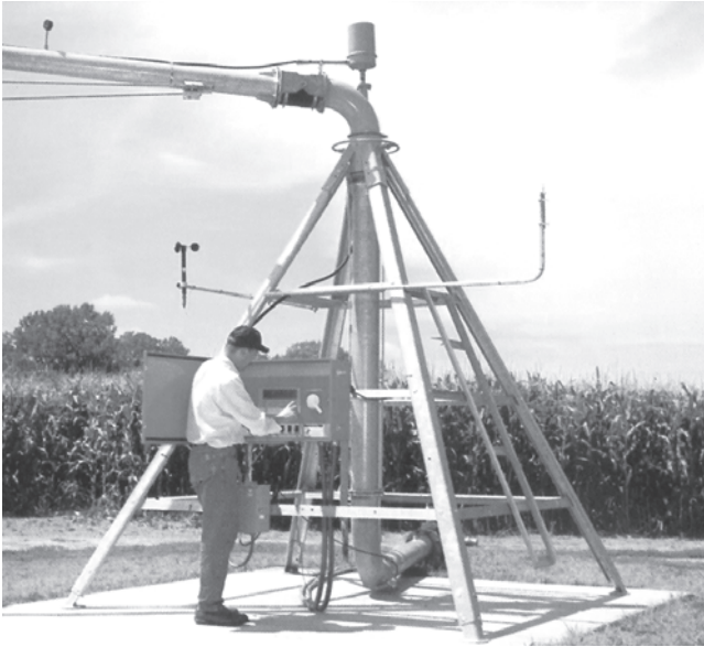
FIGURE 10.4 - The Central tower and the control panel.
