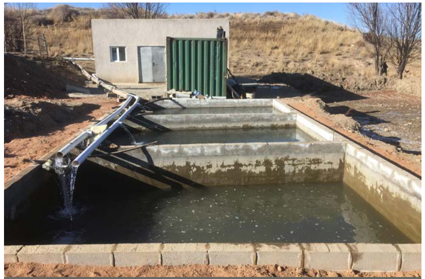
Water inlet supply and hatchery building
