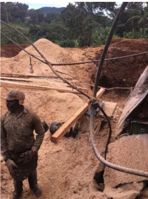
Figure 5: Electrical cables hanging all over the sawmill
