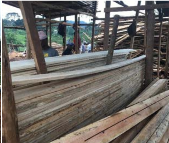
Figure 8: Unstable stacking of timber
