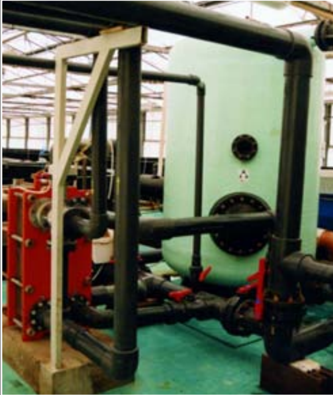
Fig. 65 - Pressure biofilter and plate heat exchanger
