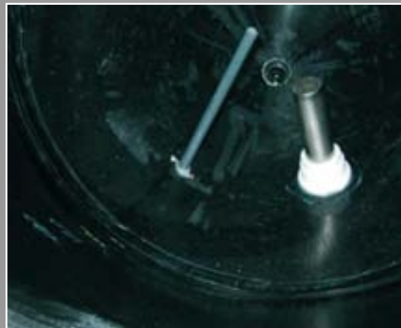
Fig. 84 - Internal view of tanks in Fig. 83: the heater and the thermostat probe
