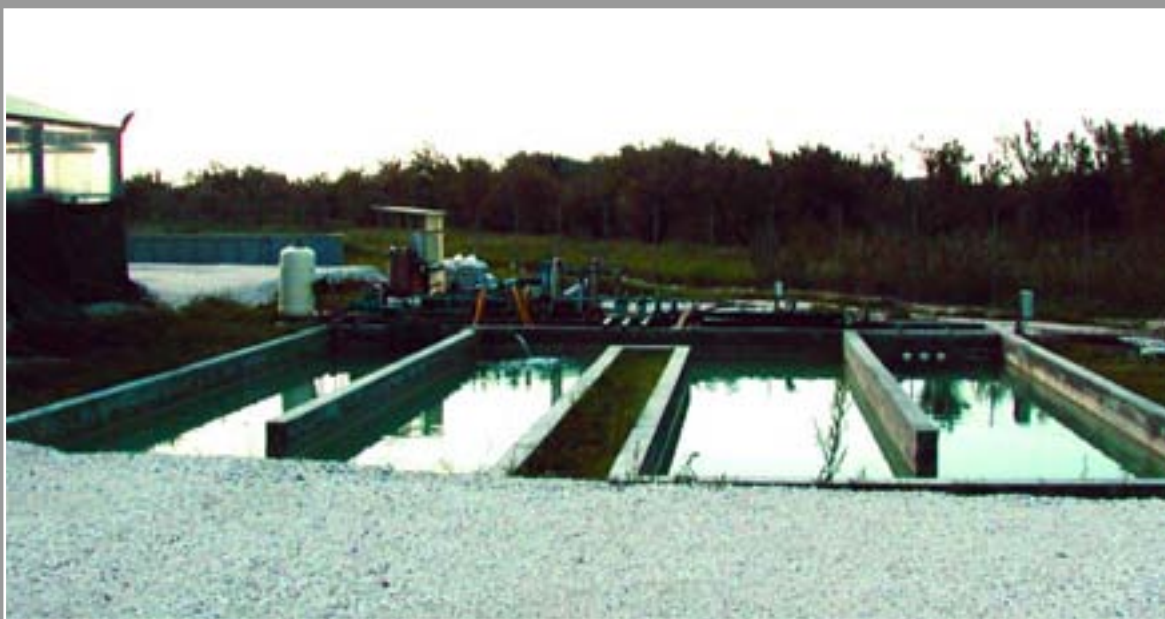
Fig. 69 - Concrete settlement tank
