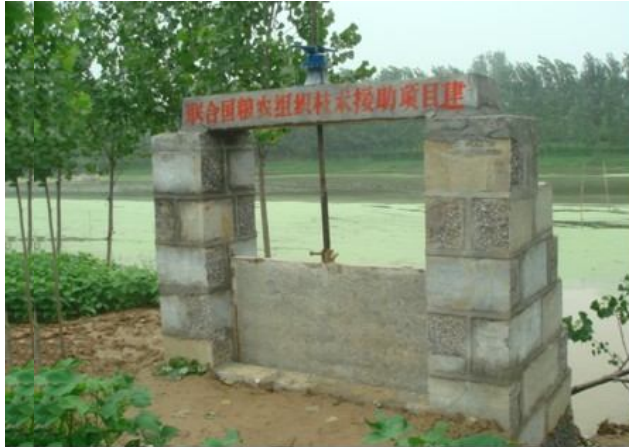
Photo 3-3-1: Sluice gate of the Drainage Culvert in Liuxi (photo by Wang Yanguai)
