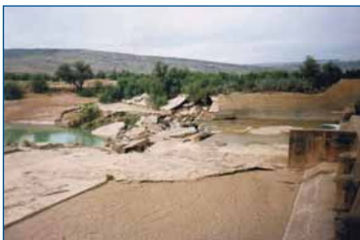
FIGURE 7.5 Diversion weir blown up by farmers as it interfered with the base flows, Pakistan
