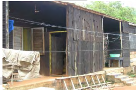
Timber houses in a poor state
