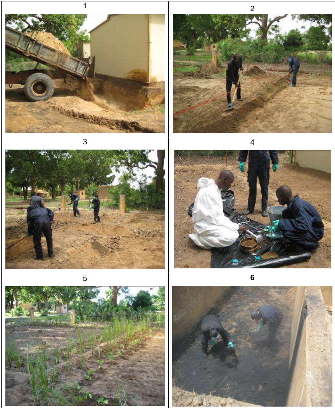
FIGURE 3 Implementation of risk reduction in Molodo. 1) Filling of the excavated center with biological active soil. 2) Making elevations around the landfarm. 3) Mixing the first charge on the landfarm. 4) Sampling on the landfarm. 5) Vegetation on the center area and around the landfarm. 6) Enrichment of soil in the concrete construction with charcoal.
