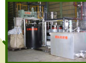
⑤ Pyrolysis (Sludge)
