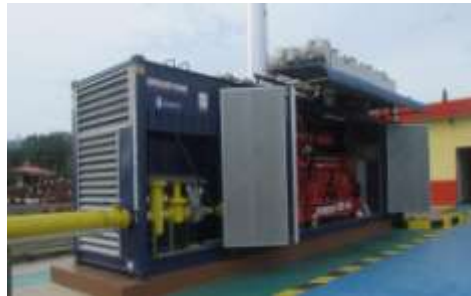
GAS ENGINE FOR ELECTRICITY GENERATION
