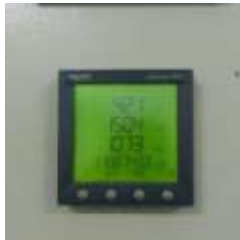
Kwh METER (ELECTRICITY GENERATION)
