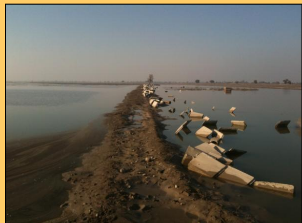
Watercourses damaged by the floods in Village Bubak, District Jamshoro, Sindh.
