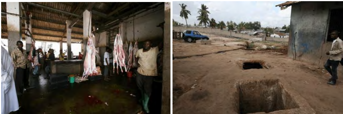
Figure 14: The Ilala Municipality slaughterhouse in Dar es Salaam: broken dressing shelf and main drainage system, October 2012
