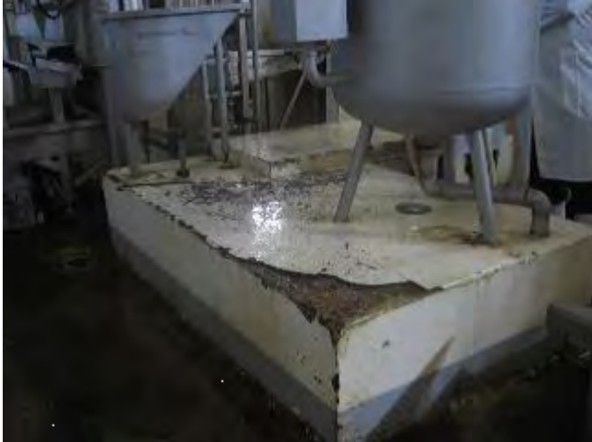
Figure 2: Cracked and peeling concrete in an export slaughter facility after four years of use, September 2012
