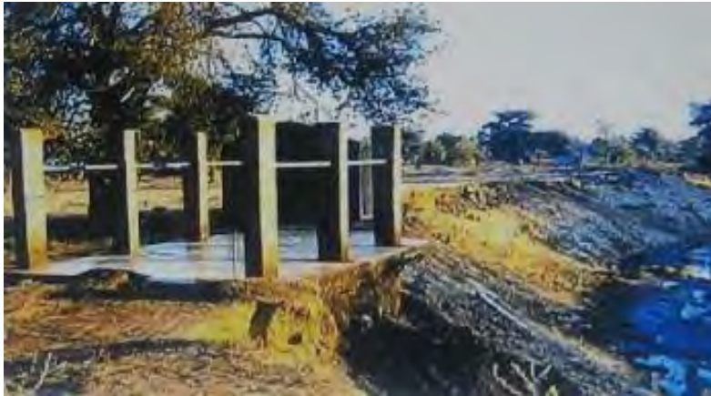
Figure 9: Dilapidated slaughter slab in the Usangu Plains, ideally situated to dispose of waste in the watercourse, 1998
