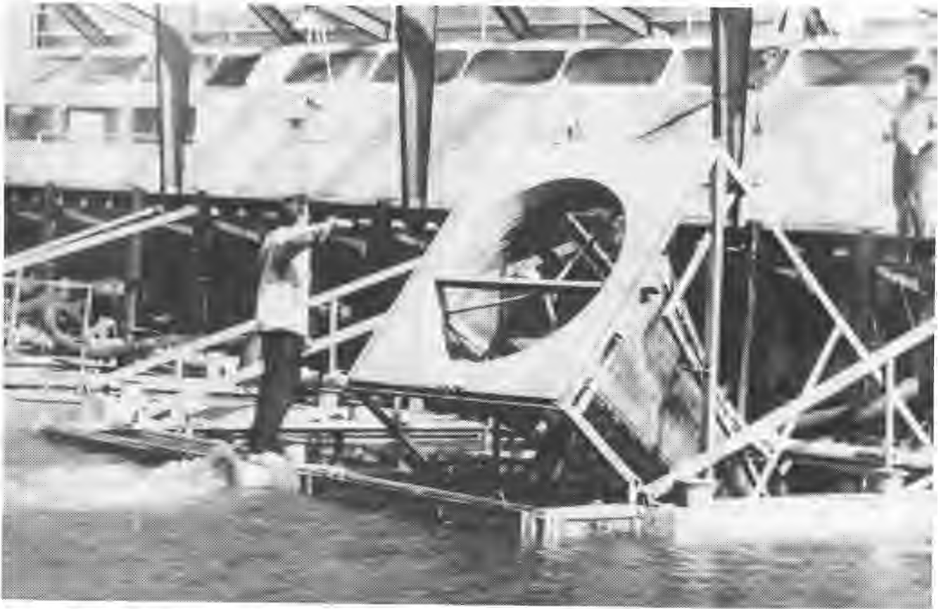
Plate 8. Vertical panel V-screens with a fish-diverting device in each section.
