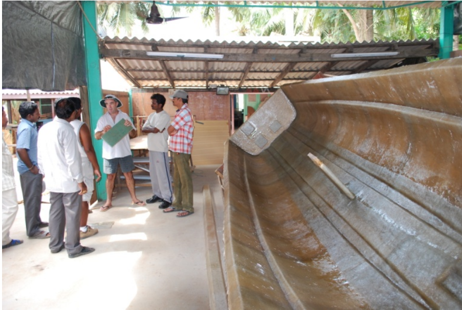
Figure 20. Training in FRP boat building in Kakinada, Andhra Pradesh, India (Photo: BOBP-IGO)
