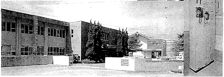
▲ハイテク室 虚空蔵山中継局向1.5GHz帯多重回線架 Hi-Tech Room Multiple Radiotelephone Equipment for Kokuzozan Transmitting Station
