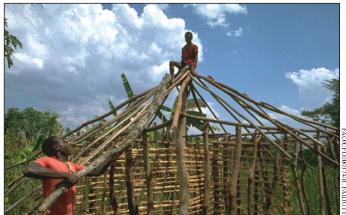
The second version of Uganda's poverty reduction strategy lists forestry as an urgent short-term priority for funding (house construction with Ficus wood)
