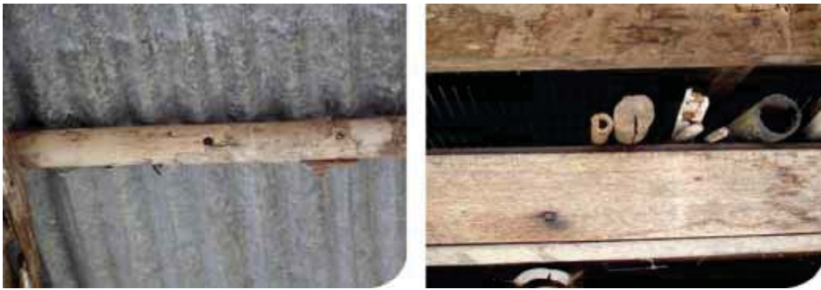
Figure 2. 9. E Nests of solitary bees in roof beams and structures provided for nesting.
