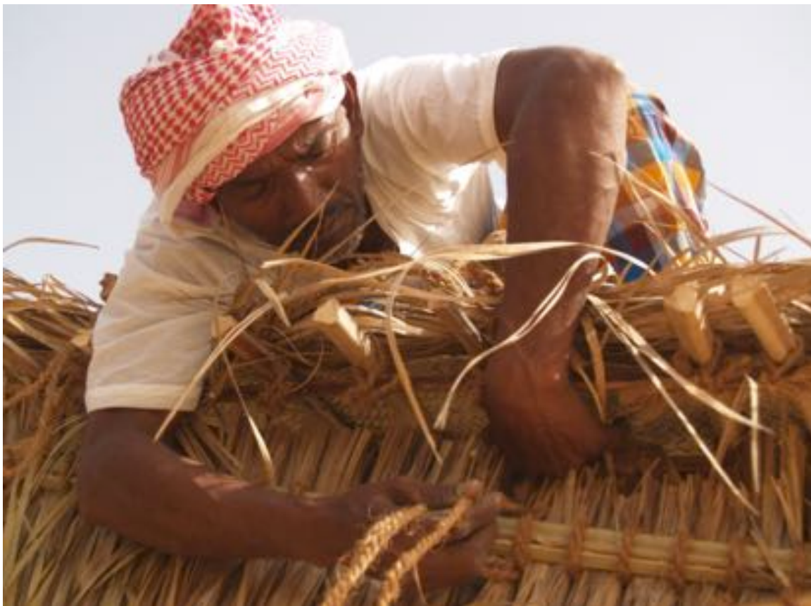
Figure 13. Fastening the roof of a date palm leaf house to the cross beams and external palm panels, using rope made of palm hair derived from the top of the date palm's trunk (Source: Rhawker's Blog https://rhawker.files.wordpress.com/2011/06/p1010949.jpg )
