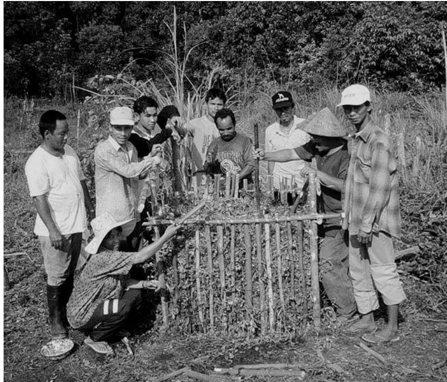
Photo. Final stages in construction of a compost bin in East Kalimantan (Borneo), Indonesia by IPM farmer participants. A plastic covering was later added to protect the compost from rainfall. Ingredients included local succulent weeds, cow dung and lime.
