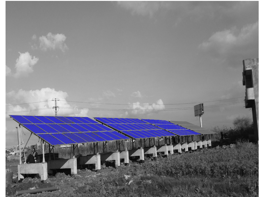
Al-Afir project – Solar powered irrigation system in the Nile Delta.
