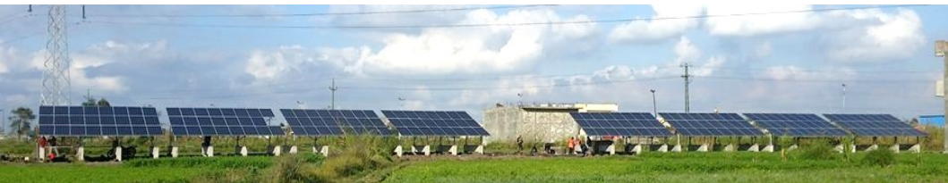
Al-Afir project – Solar powered irrigation system in the Nile Delta | Source: FAO, 2017, El- Behiera Governorate, Egypt
