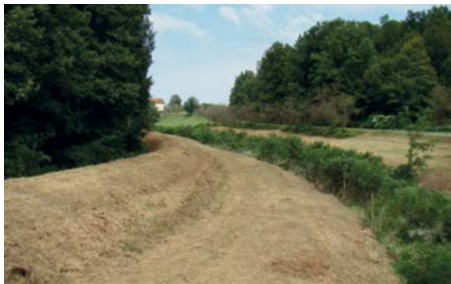
Circumferential (diversion or interception) canals to protect the agricultural area in the plain from mountain waters, Nožičko, Srbac municipality, north Republic of Srpska.
