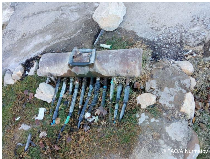
Picture: Chuya village (Navoi /Nurota) Handmade leaky vessel-based construction of drinking water pipes used for main street tree irrigation and households supply (November 2021)
