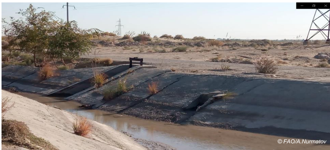
Picture: Canal in Bukhara, Sayot water station: Broad and long cracks (visible with the plants) in the concrete leading to leakage to the underground and sediments that undermine the water flow.2021
