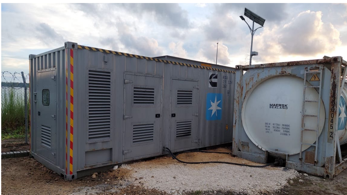
FIGURE 20: GENERATOR AND ISO FUEL TANK
