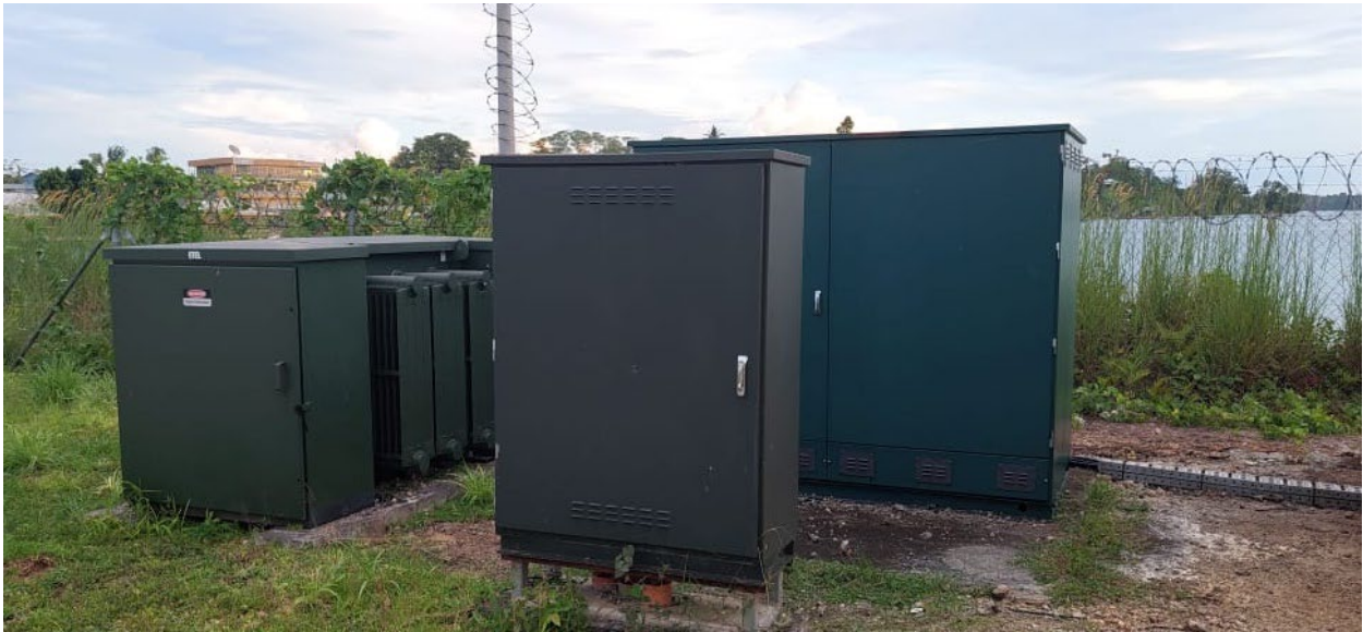
FIGURE 21: BREAKER UNITS CONNECTED TO GENERATOR AND PLUG IN YARD
