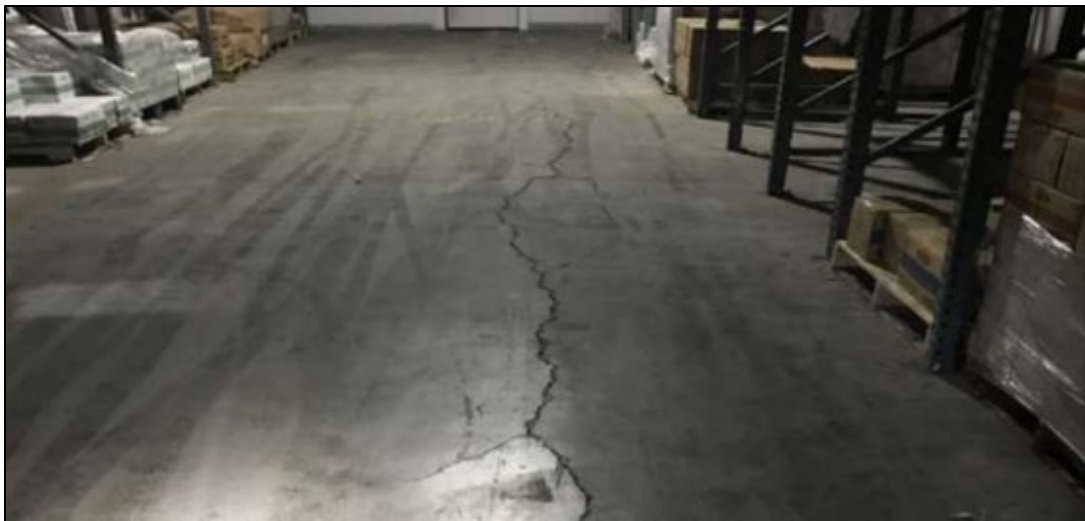
Figure 23. Frost heaving on a cold room floor
