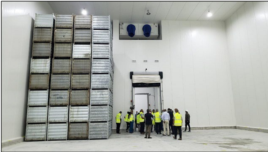
Figure 9. Inside one of the cold rooms at the CCCS Seychelles
