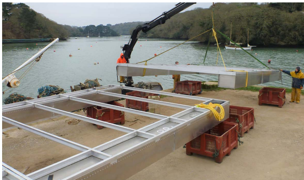
FIGURE 5.21 Lifting the two halves of the Flupsy into the water using a crane
