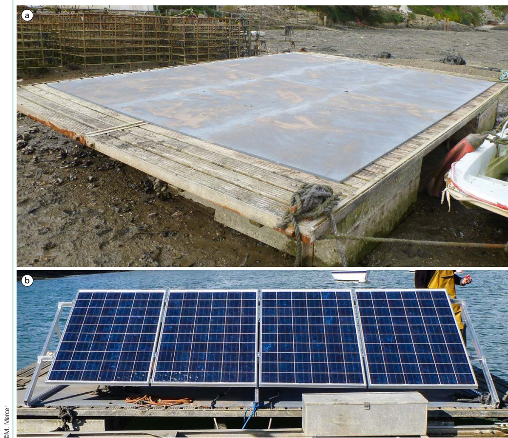
FIGURE 5.32 (a) Solar raft. (b) Solar raft with panels installed
