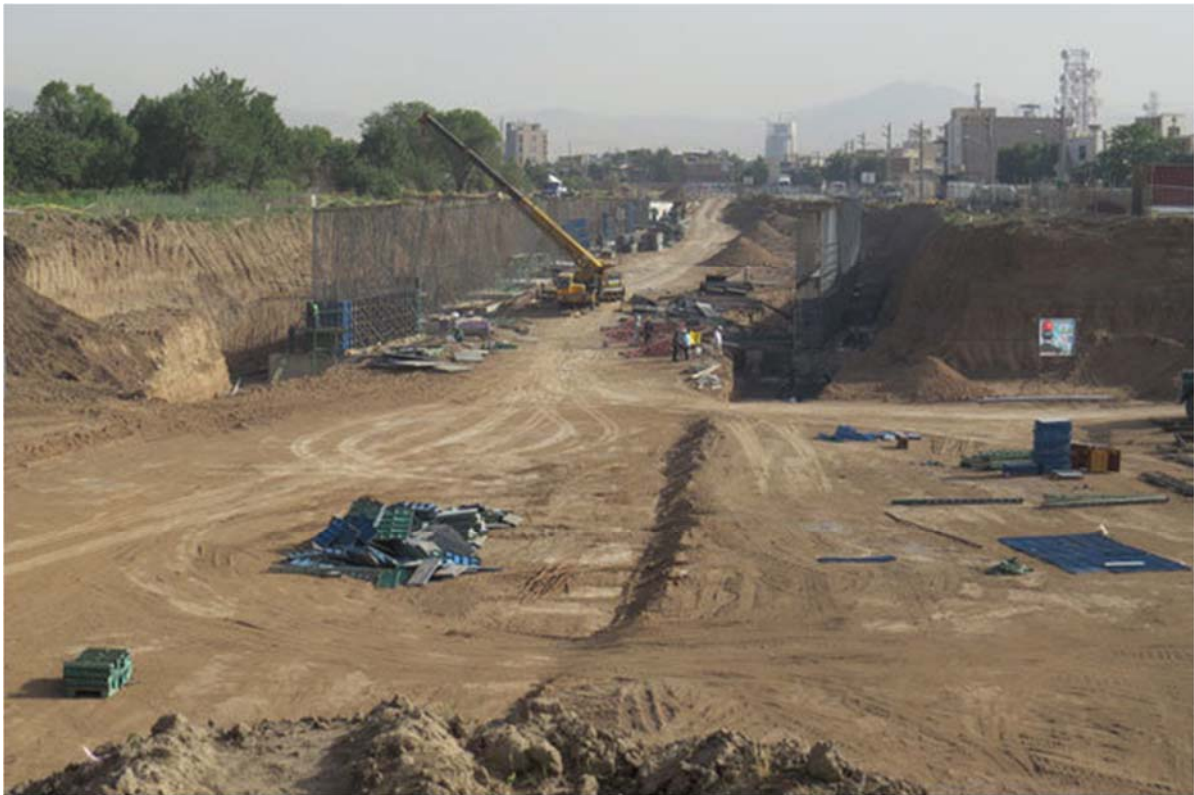
Figure 15: Deep cutting of Bāghestān soil during the construction of a bridge; photo by ASCL NGO
