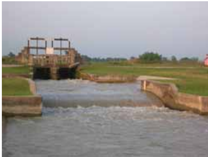
Plate 28 Head of secondary canal equipped with a measurement device (gauge) of very low accuracy (Nepal).
