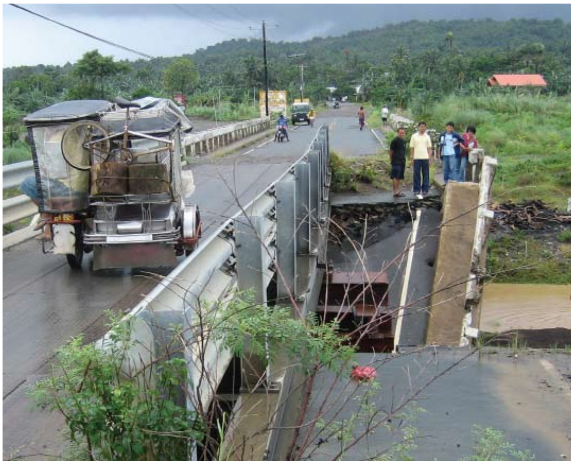
Makeshift bridge still serves the General Santos community since the floods of 2005
