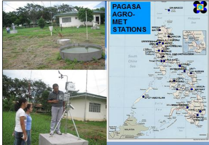
Figure 12 Automatic weather station being installed at PAGASA Weather Station in BUCAF, Guinobatan, Albay on August 2010
