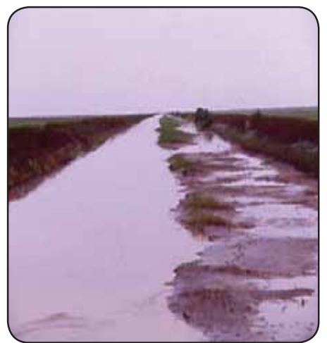
Photo 7: Canal Siltation Sudan
