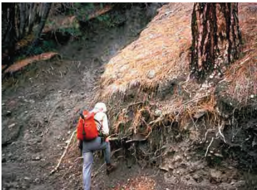
Figure 2.4. Ponderosa pine tree buttressing a slope above a forest road. The unprotected portion of road cut to the left has failed. Mendocino National Forest, California, 1978
