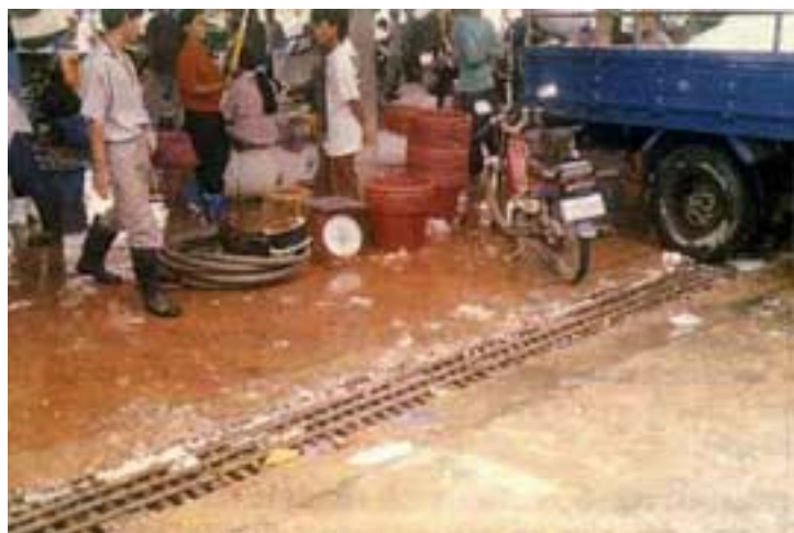
Drain for waste water from landing/cleaning pier at the FMO Port, Phuket
