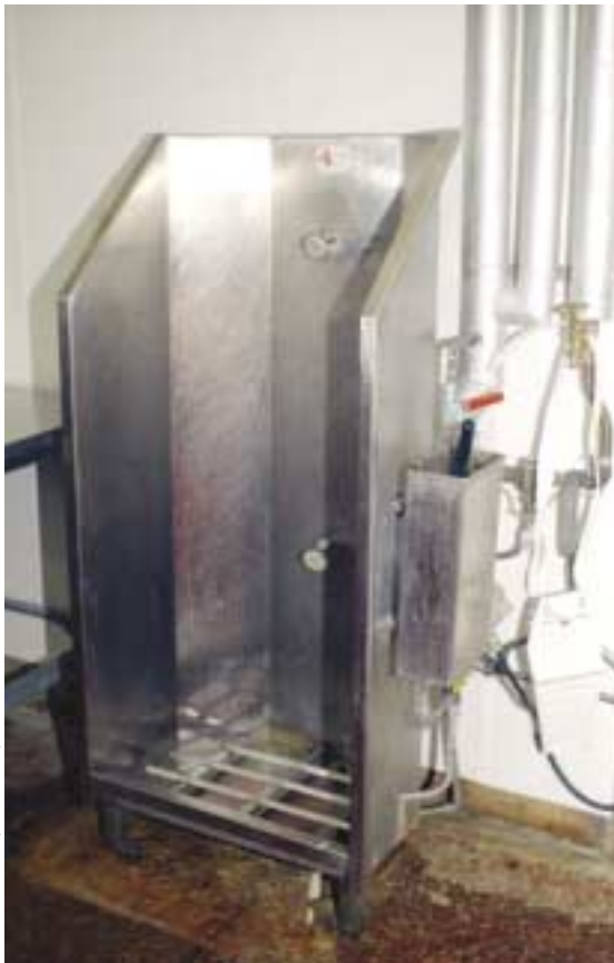
PHOTO 10.1 GOOD PRACTICE: stainless steel apron wash with knife sterilizer
