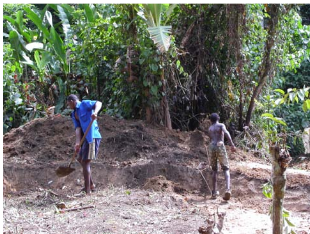
Figure 5: Most ponds are hand dug. Although most claim to use “cut-and-fill” technology, inevitably the dirt is heaped at the closest location and rarely compacted. The result is a leaky pond with too much levee on the shallow side and too little on the deep end (Cameroon).
