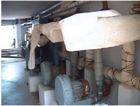
Filter bags for the air blower are kept clean
