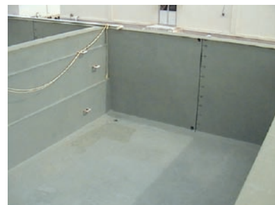
These tanks are painted with epoxy and well maintained but their corners should be rounded to allow easy cleaning and efficient disinfecting during preparation
