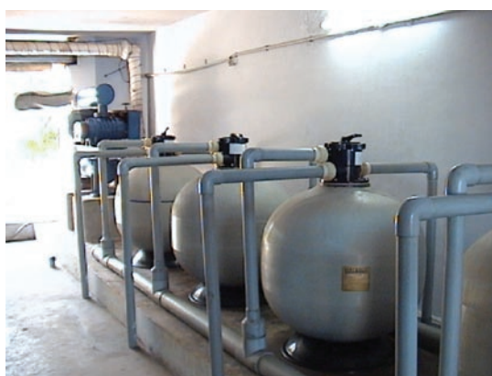
Recirculating sand filters (RSF) are properly maintained at some hatcheries
