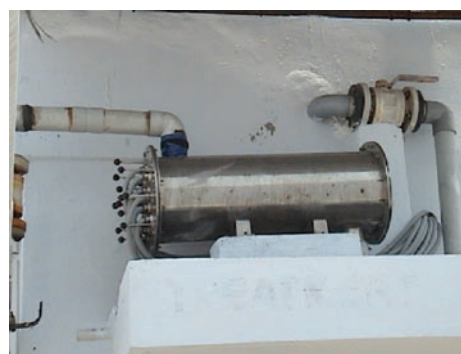
Wipers are installed to clean the UV lamp at some hatcheries
