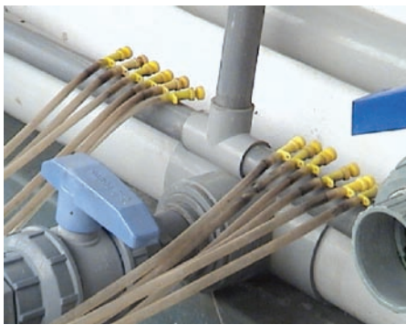
Air distribution pipes and diffusers should be cleaned, disinfected regularly and replaced when the pipes become contaminated (below, Tamil Nadu) The dark coloration at the connection and valve indicates the presence of dirt in the air supply and also inadequate cleaning of the air supply system
