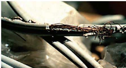
damage to cable
