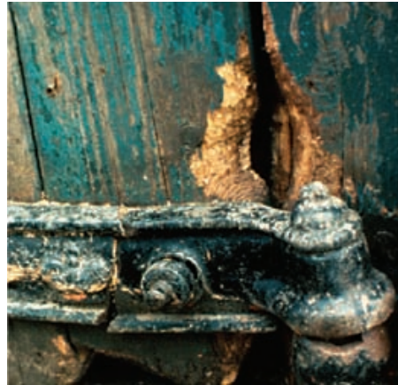
damage to structures
