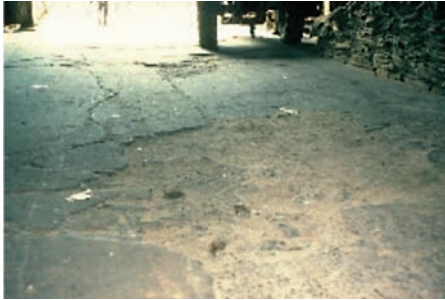
FIGURE 4 Badly broken floor allows dust and insects to accumulate
