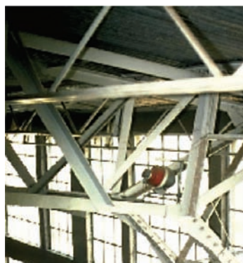
FIGURE 21 A space sprayer in position on the roof lintel
