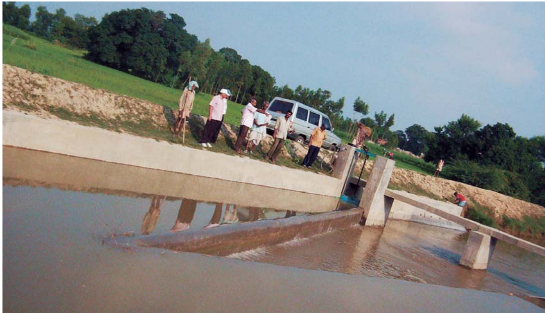
Plate 2. Duckbill weir at Tikri distributary
