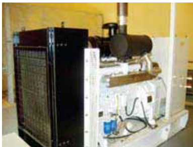
One of three 100 kW dutch generators at Garalo able to run on Jatropha oil, diesel or a blend (Photo: Smail Khennas)
