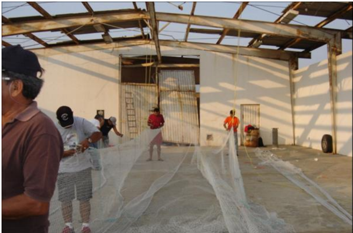
Preparation of side, upper and lower panels for hanging of lateral ropes
