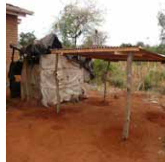
The purpose of our mission: to replace the often dangerous and decrepit cooking shelters with new, secure, structures.
